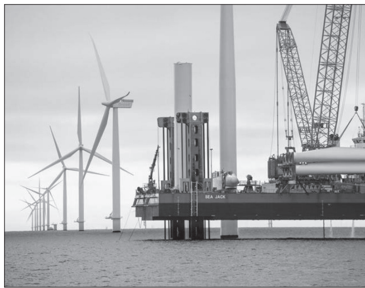
A lift boat installs the base of a wind turbine at the Anholt Offshore Wind Farm off the coast of Denmark in 2013. Courtesy of Orsted
