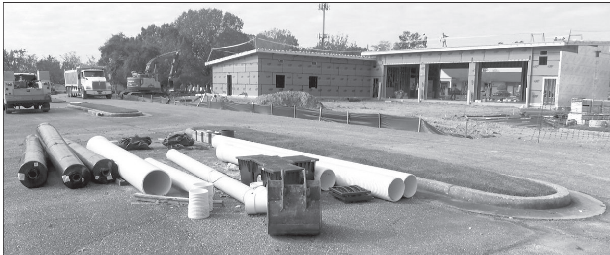
The future site of East Baton Rouge EMS Station No. 9 takes shape along Airline Highway. The $2.6 million facility, set to open in May 2025, will enhance emergency response times and serve as a disaster supply hub.
