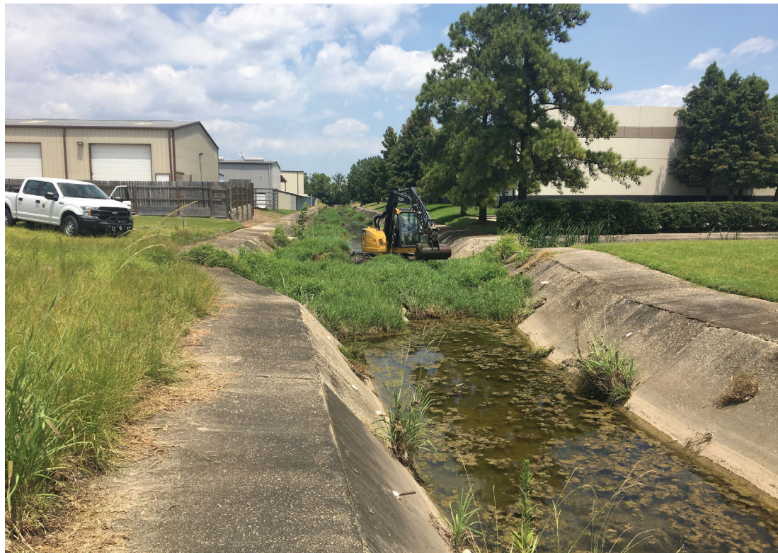
The Department of Public Works is making progress on two drainage improvement projects in the city-parish. (Source: Office of Mayor-President Sharon Weston Broome)
