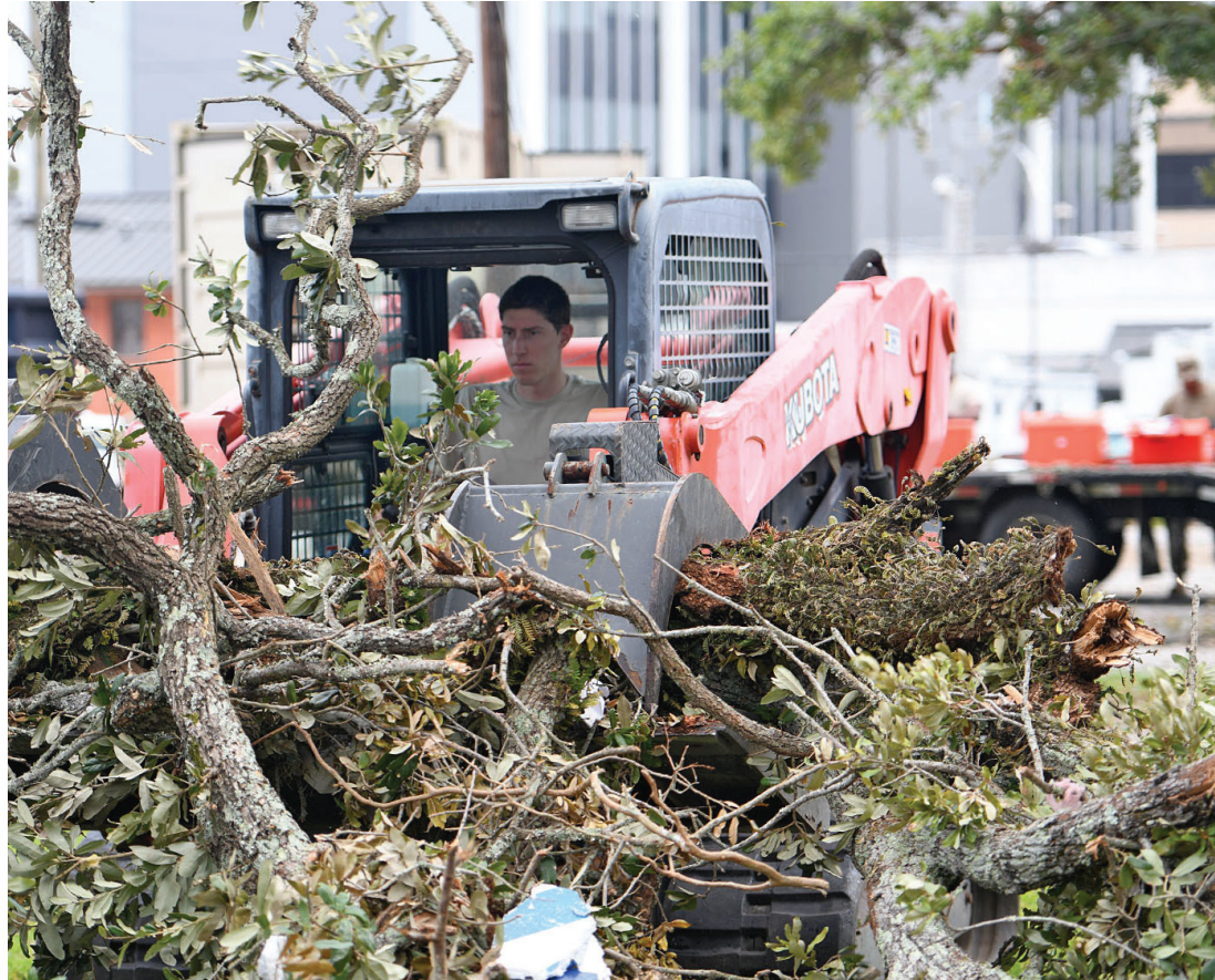
Louisiana National Guard Senior Airman William Bommer, 159th Civil Engineering Squadron's heavy equipment journeyman, removes tree branches in downtown Lake Charles, La., Aug. 30, 2020, after Hurricane Laura caused heavy damage in the area.
